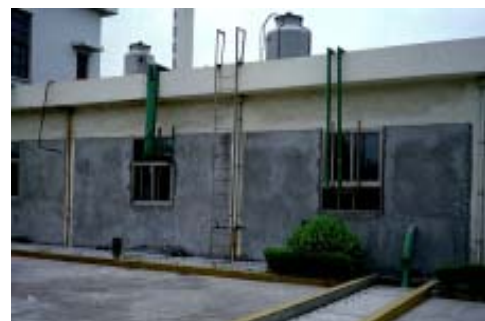
Noise-proof wall added to air compressor room (Jiangsu Mabuchi)
