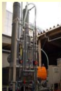
Ground water pumping and purification system
