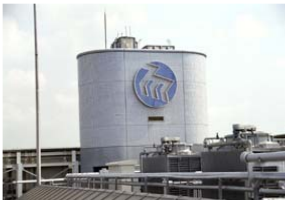
Reused water (rainwater) tower installed on the top of the building of Headquarters
