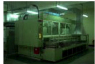
Hydrocarbon scrubber introduced in fiscal year 2003 (Hong Kong Mabuchi)
