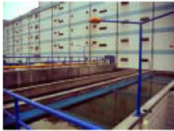
Wastewater treatment facility constructed in Guangdong Factory 1 (Hong Kong Mabuchi)
