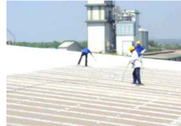
Thermal insulating paint being applied to the factory roof of Vietnam Mabuchi (in fiscal year 2004)
