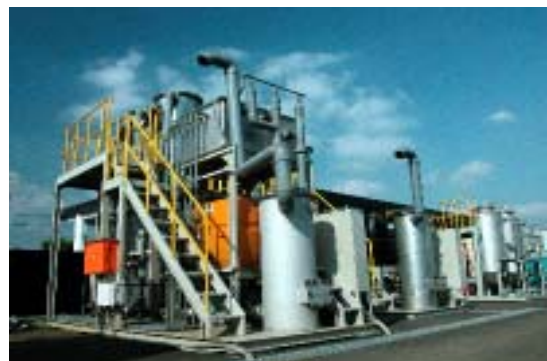
Groundwater decontamination facilities at the new site of Mabuchi Motor's Headquarters
