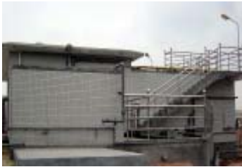
Construction of waste water treatment facilities (with a treatment capacity of 200 tons per day) at Dongguan Mabuchi was completed in August 2004.
