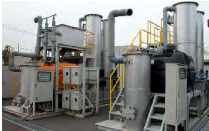
Soil decontamination facilities installed at Mabuchi Head Office
