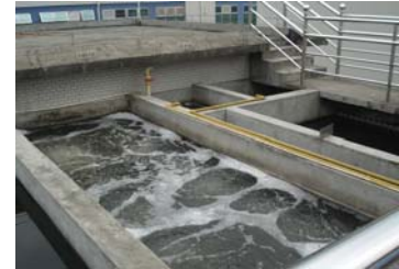
Simplified wastewater treatment equipment
