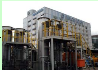
The water pumping and aeration equipment installed in the premises of Mabuchi Motor Head Office.
