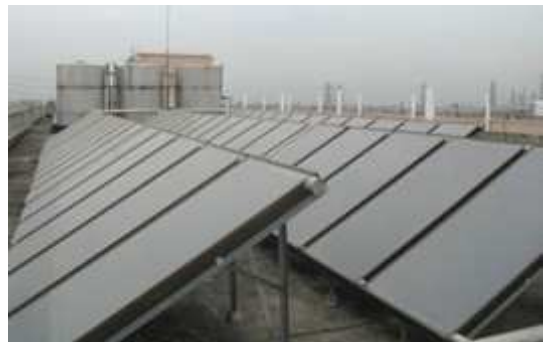
A solar water heater installed on the roof of the company dormitory
