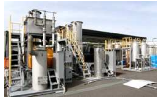
Soil decontamination equipment installed in the premises of the Head Office
