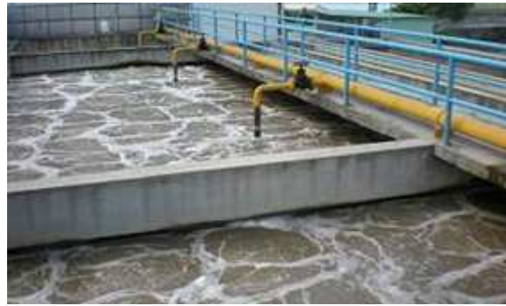
Treatment tank for domestic wastewater
