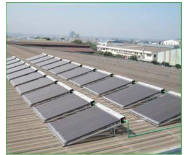
We used less gas to heat water because we now have a solar water heater installed on the roof. (Vietnam Mabuchi)
