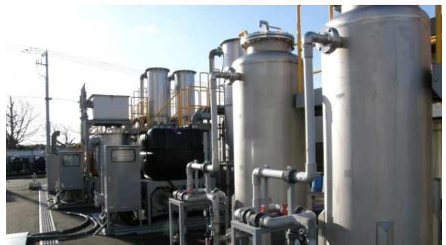
Soil decontamination equipment installed in the premises of the Head Office
