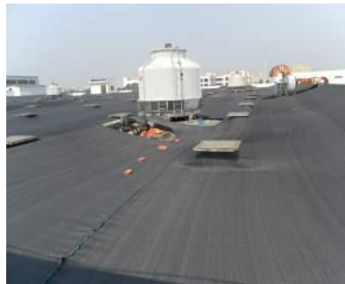
Owing to the thermal shield constructed on the roof, the room temperature in the summer was down 36% compared with previous years, and this meant we needed considerably less electricity for air conditioning. (Jiangsu Mabuchi)
