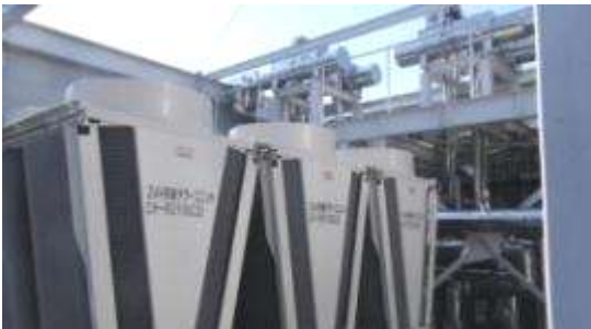
Newly introduced 24H type of heat supply system (Head Office's Technology Center)
