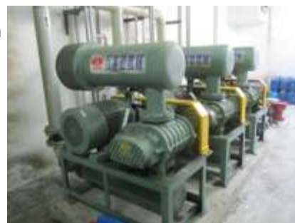
Wastewater treatment system installed in the plant
