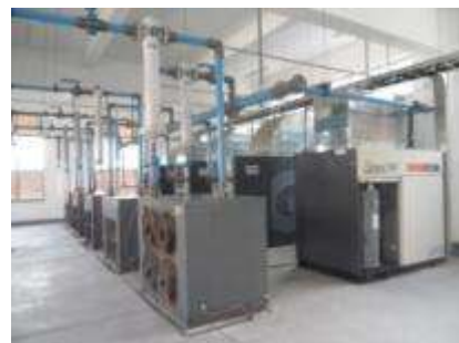
Automatic controlled compressor system
