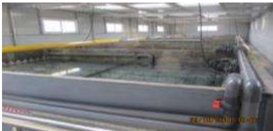
Sewage treatment system (Wafangdian Mabuchi)
