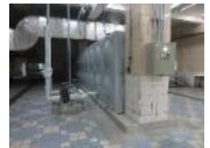
Hot water tank circulation unit
