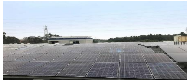
Solar panels installed on the roof
