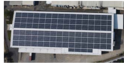
Solar power generation system installed in Danang Mabuchi
