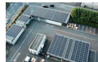
The solar power generation system installed at the Headquarters
