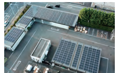
The solar power generation system installed at the Headquarters
